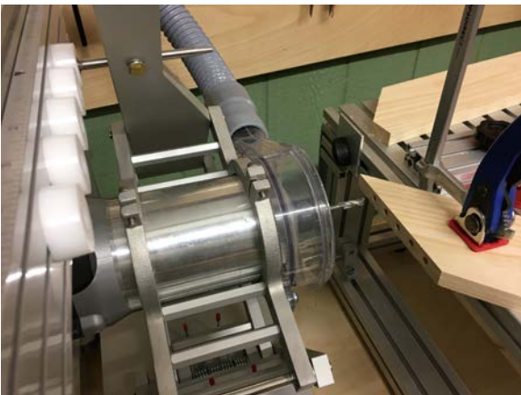
Horizontally bore holes in each of the mitered faces to be joined together
